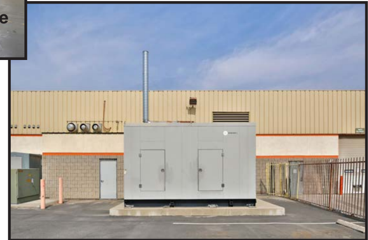
Back up Diesel Generator
